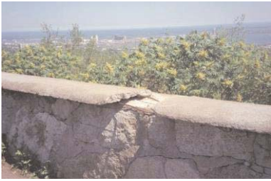
This rock wall at an overlook near 28th Ave. W. is deteriorating.
