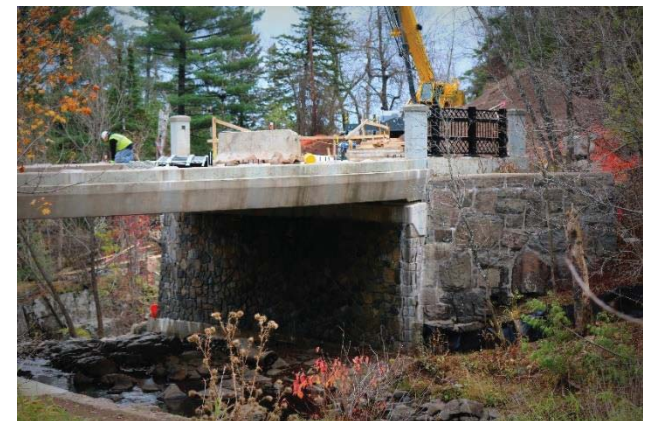
Improvements seen in the interactive map tool include on-gong improvements to the Chester Creek Bridge
